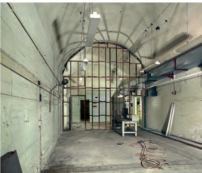
The Tape Relay Centre with the Signals Centre in the RSG at Dover Castle. Photo Nick Catford
